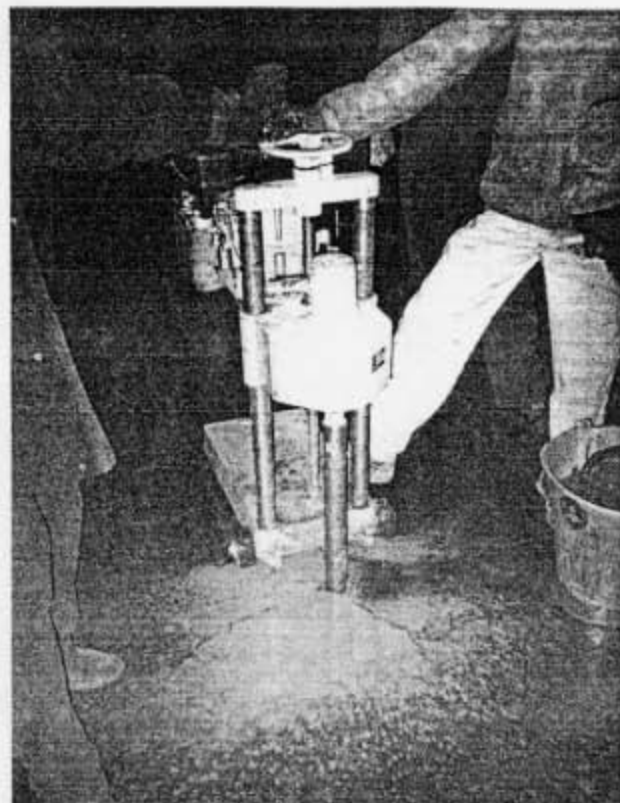
FIG. 3(b). Crack Repaired by Cutting 50 mm (2 in.) Diameter Holes at 0.61 m (2 ft) Center to Center Spacing and Subsequently Filling with Asphalt Concrete
